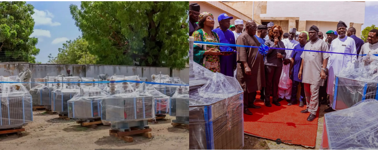
Brand-new electricity transformers, still factory-wrapped, await deployment to communities across Taraba State.
